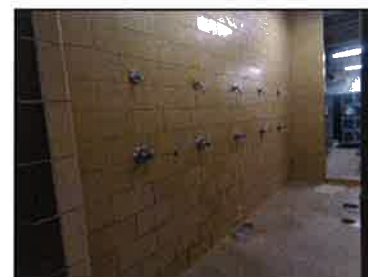
The gymnasium lockers rooms do not have a functional ventilation and exhaust system. Due to the high moisture content in these rooms, dangerous mold and bacteria strains can grow without proper ventilation
