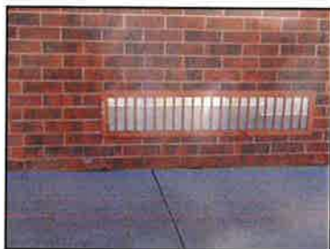
The outside air intakes of the heaters in the B building have been blocked off. This is likely because the system is undersized and cannot effectively heat the spaces with outside air.
