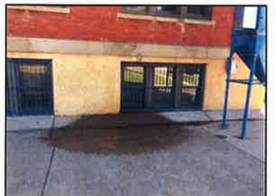
Poor site drainage
