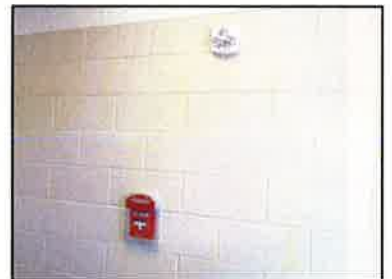
Alarm pull bar and strobe system
