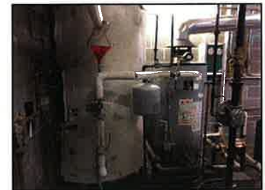
Water heater in storage tank (1974 addition)
