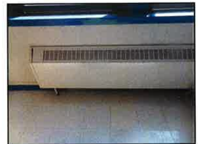
Hot water baseboard convectors heat most of classrooms and hallways in the school. The units do not provide ventilation air.
