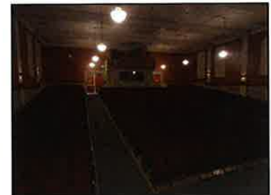
None of the spaces in the building, including the auditorium, have cooling. A packed play can become extremely uncomfortable without proper cooling.
