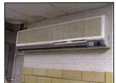
Ductless mini-split serving office areas
