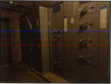
Main Distribution Panel
