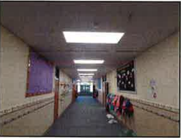
The 1964 wing has carpet floors, cmu block walls, and acoustic tile ceilings.
