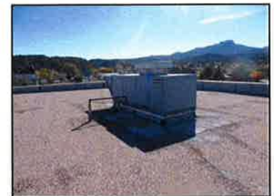
The rooftop furnace serving the gymnasium is at the end of its reliable lifespan and is due for replacement. (2002)
