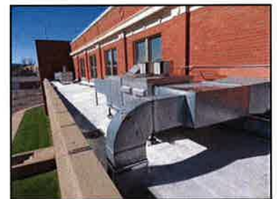
The 1922 gymnasium and lockers rooms are conditioned by rooftop furnaces that are in poor condition. The building does not have any cooling.
