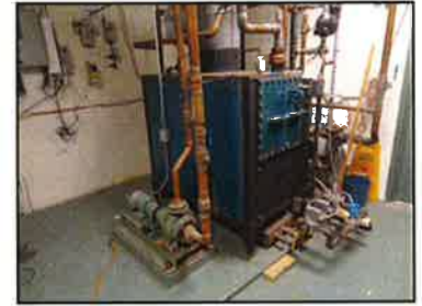
The boiler serving the hot water loop in the 1964 wing is over 25 years old. It is at the end of its recommended lifespan.
