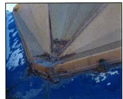
The dome is composed of aluminum panels which expand and contract throughout the year. Consequently, cracks form in the caulking between panel joints and leaks develop every year.
