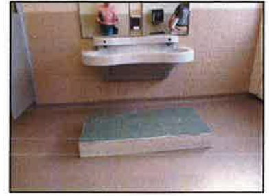
Bathroom accessibility issue
