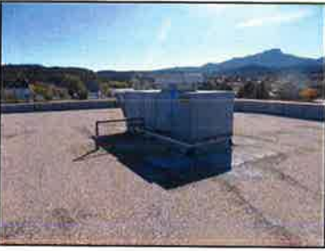
The packaged rooftop units serving the 2002 spaces are over 15 years old. They are due for replacement.
