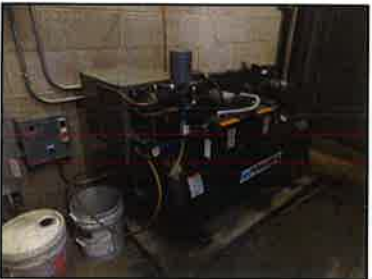
Air compressor for pneumatic controls
