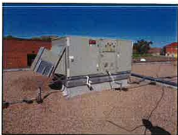
The High School A building is conditioned by packaged gas/dx rooftop units. The units were installed in 2012 and are in good condition.
