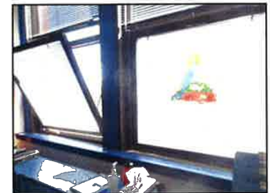
The 1911 Middle School received double pane aluminum frame windows over 25 years ago. Many of the window frames are in poor condition and can no longer open.
