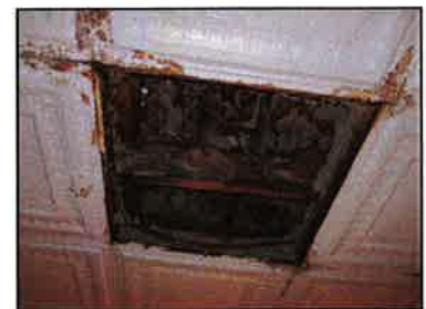
Water-damaged ceiling joists above auditorium
