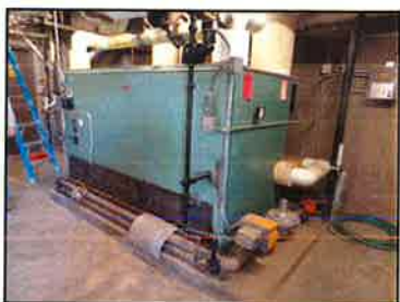
The B building is conditioned by hot water cabinet heaters. The boiler serving the hot water loop is in poor condition and is at the end of its reliable lifespan. The building has no cooling and poor ventilation
