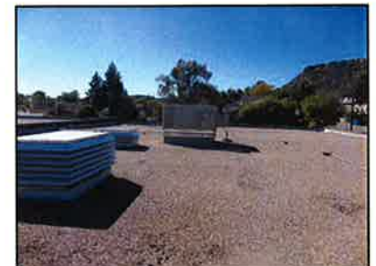
The ballasted built-up roof atop the High School A building is in adequate condition. The roof atop the High School B building is in poor condition and due for replacement.
