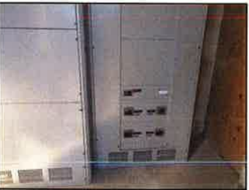
The new main distribution panel installed in 2002. It is in excellent condition and is providing the building with sufficient electrical capacity.
