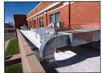
The 1922 gymnasium and lockers rooms are conditioned by rooftop furnaces that are in poor condition. The building does not have any cooling.
