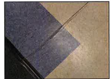
The settling slab has also produced a wide array of cracks in the floor.
