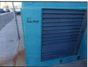
The generator was installed in 1993 and has been unreliable for the district. It was unable to start during the most recent power outage.
