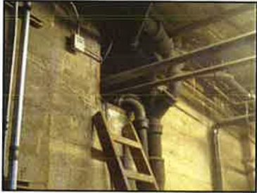
The underlying foundation walls still appear to be in good condition in the few areas where they could easily be seen
