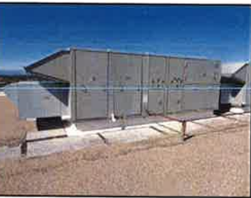
The rooftop units at Fishers Peak are over 15 years old. The district should budget for their replacement in the next 1 to 3 years.
