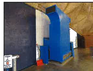
Large hot water air handlers located around the stadium perimeter heat the facility. There is no cooling in the building.
