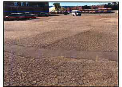
Typical deteriorated parking lot & asphalt conditions
