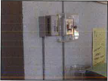
Ineffective pneumatic controls
