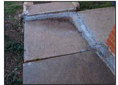
Exterior settling and cracking
