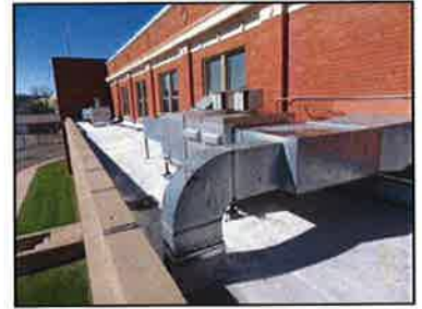
Dilapidated rooftop furnaces heat the 1922 gymnasium. They have reached the end of their serviceable life.
