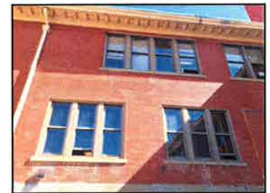
Windows are typically propped open for outdoor air to combat comfort issues
