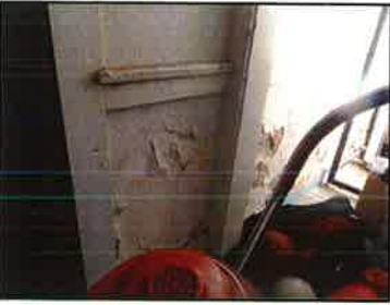
Water is infiltrating the below grade walls in the 1911 and 1922 buildings causing damage to interior finishes
