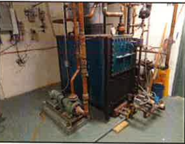
The boiler serving the Eckhart cafeteria is in poor condition and is due for retirement. A single gas/DX rooftop unit should be installed above the cafeteria to provide heating and cooling.
