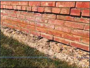
Signs of exterior foundational decomposition
