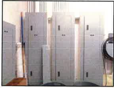
The electrical distribution in the building is in good condition. The MDP was sized properly and the classrooms have an appropriate number of outlets.
