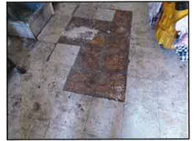
The subfloor in some of the 1911 rooms has been damaged and needs to be replaced.
