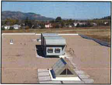
The classrooms are conditioned by packaged DX VAV air handlers located on the roof. Each room has a dedicated terminal VAV box with electric reheat.
