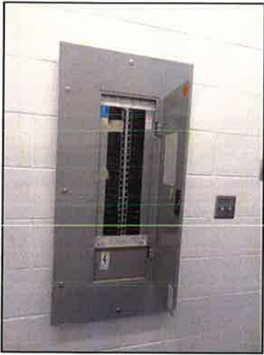
The 1911 building received an electrical upgrade in 1993. The sub-panels and main distribution panels are adequately sized and are in good condition.
