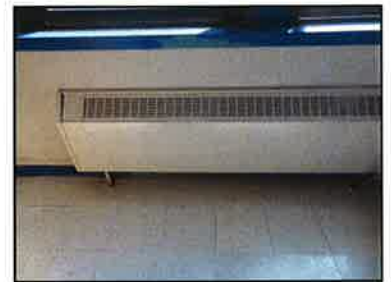
The classrooms in the 1911 building are conditioned by hot water baseboard convectors. None of the rooms have any cooling or mechanical ventilation.
