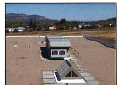
The building is protected by a ballasted built-up roof that is in fair condition. It is original to the 2002 construction.
