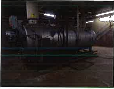
The High School Gym boilers are over forty-five years old. They are extremely inefficient and are difficult to maintain.
