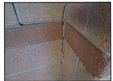
The settling of the concrete slab has damaged many of the interior walls in the school.
